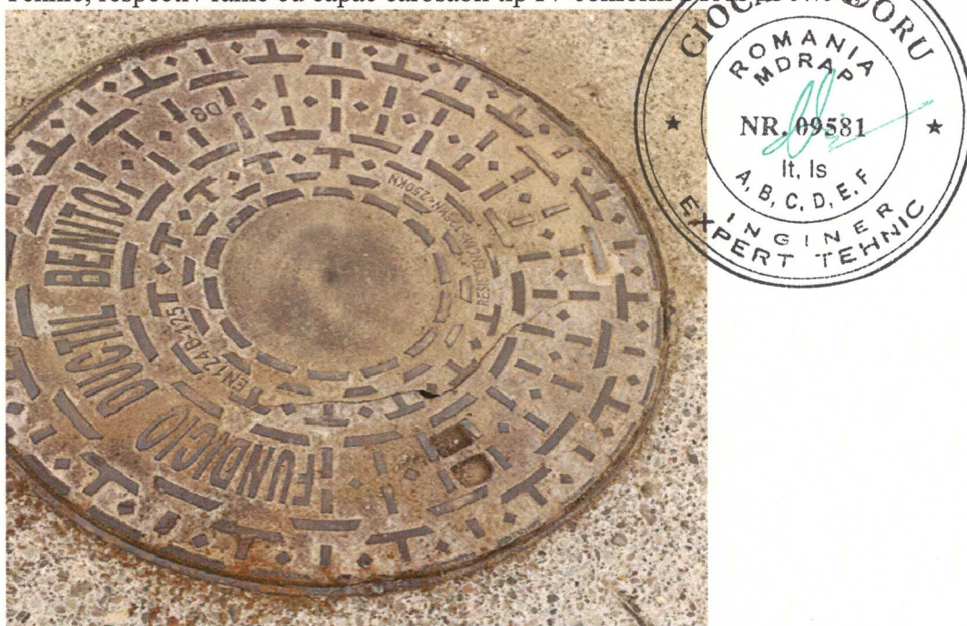
Fig. 1 Capac neconform fisurat
